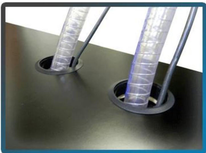
Pipe and cable management
